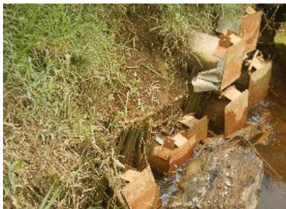
Figure 4. A poorly maintained canal outlet
