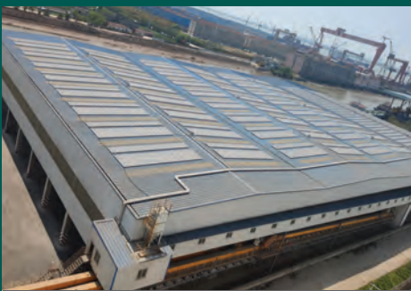
We are constructing photovoltaic power plants in all our factories in China.
