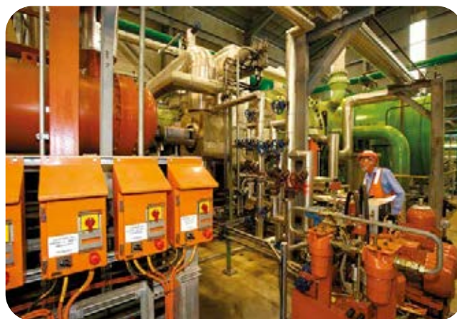
Cogeneration plant in Queensland, Australia.
